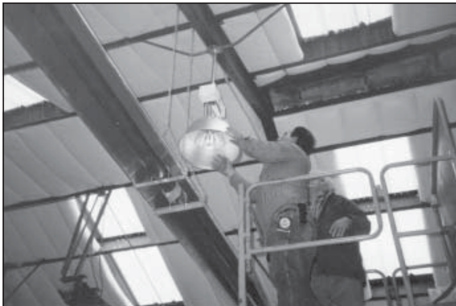
Insulation, radiant heating, skylighting and efficient lighting - Highway Department Maintenance Building. Source: ECMD
